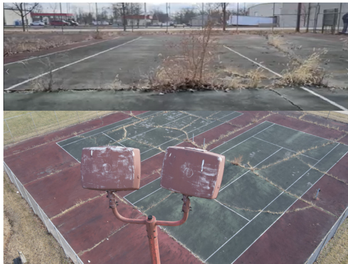
Washington Elementary Tennis Courts, Current Condition (Unplayable)
